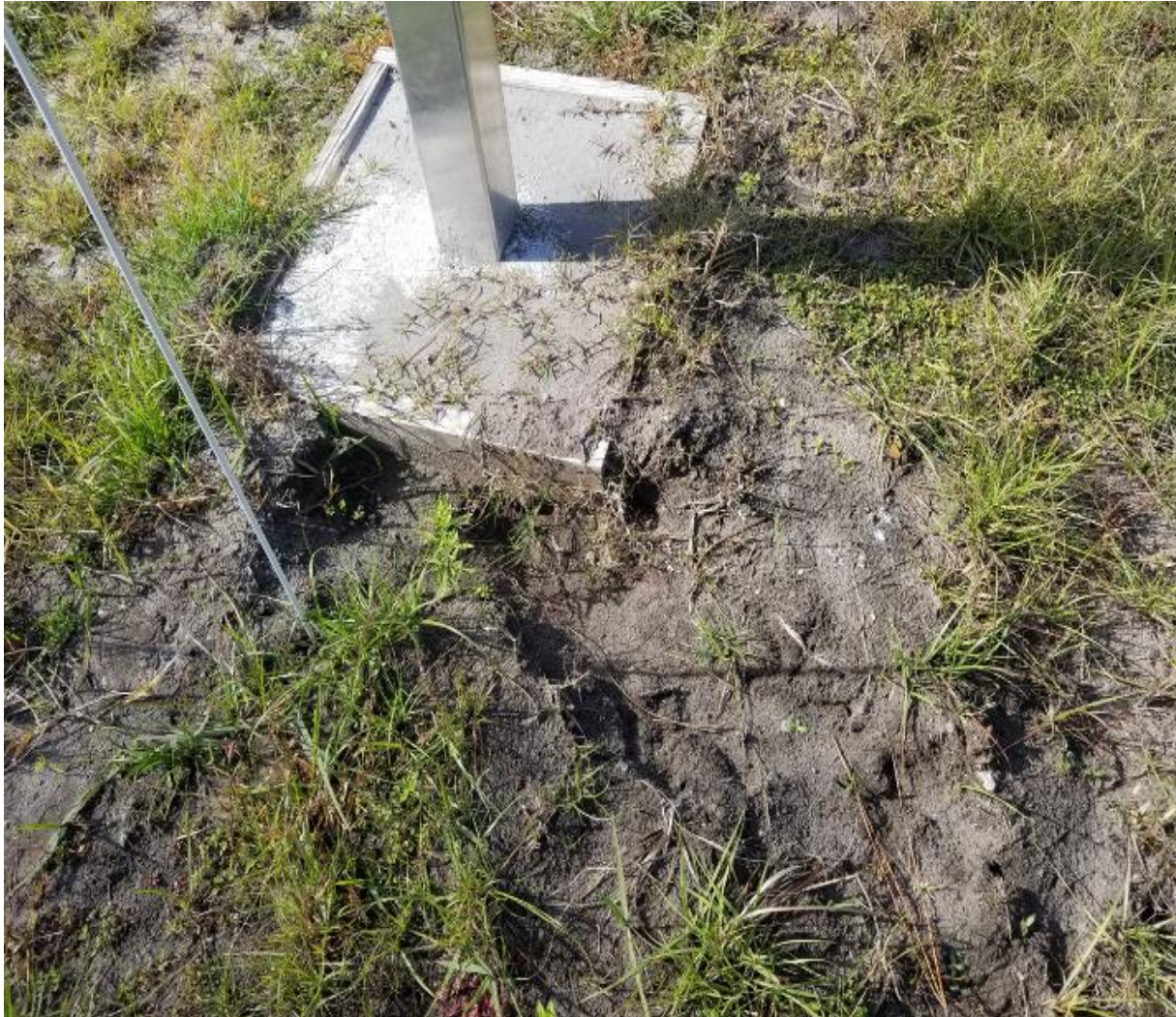
Figure 10. Erosion around LF-3's concrete pad
