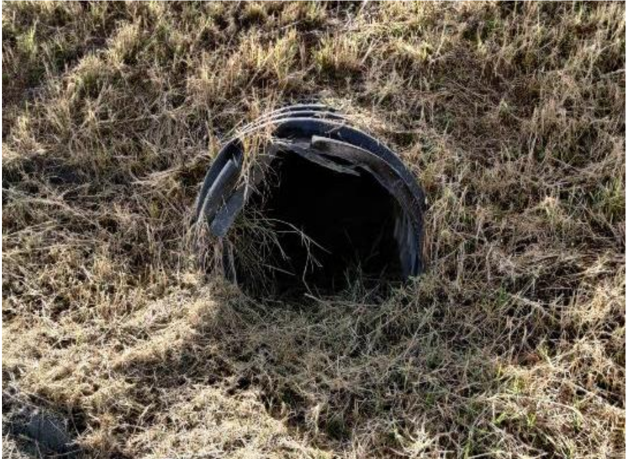
Figure 7. Thick vegetation around the Cell-4 culvert outlet
