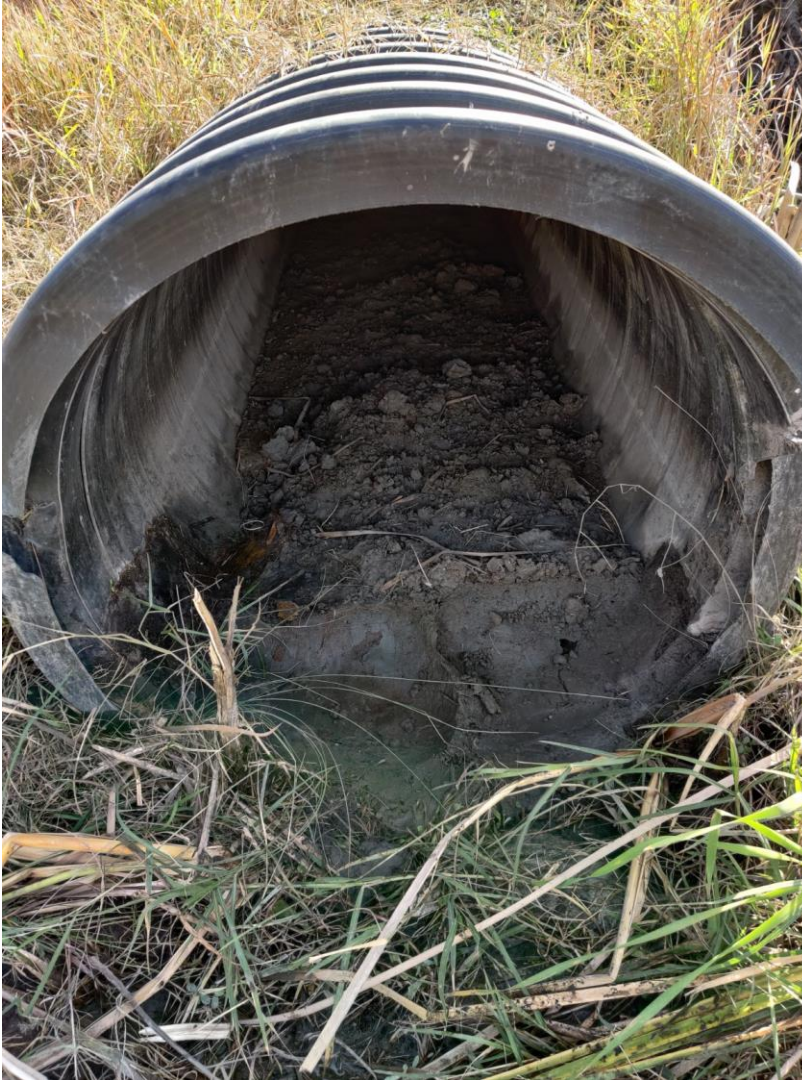
Figure 12. Sediments accumulation in one of the culverts located in the southeast corner of the landfill
