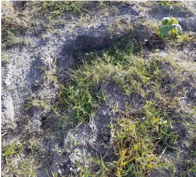
Figure 5. Erosion around the south-east corner of the Northern Ditch
