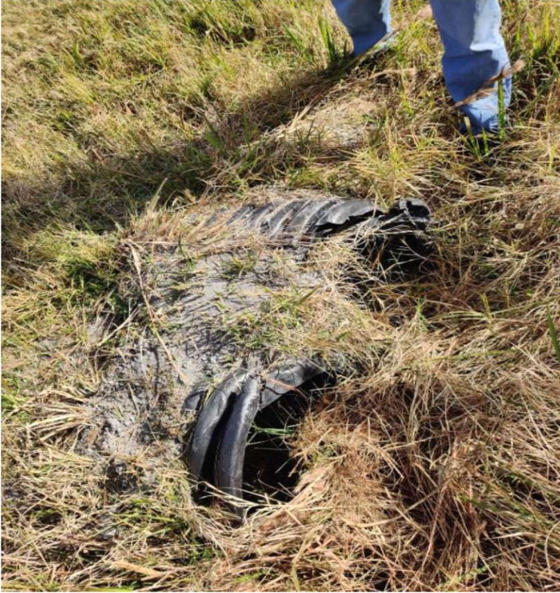
Figure 8. Thick vegetation around the Cells 3 and 4 culvert inlets
